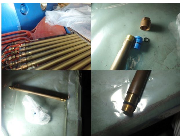
Figure 6: Feedthrough pipes of trim coils and hardening of an O-ring at C8-OUT.
