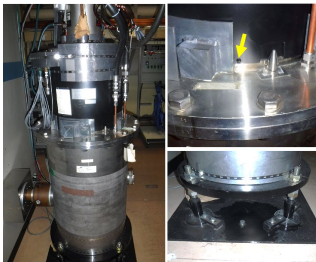
Figure 2: Water leakage from Klystron magnet.
