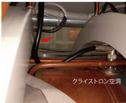
Figure 8: An RF leakage point at the RF inlet of the klystron. A schematic drawing and a photograph are shown in top and bottom, respectively. A leakage was found at a short cable to the klystron cavity as indicated by a red arrow in the bottom.
