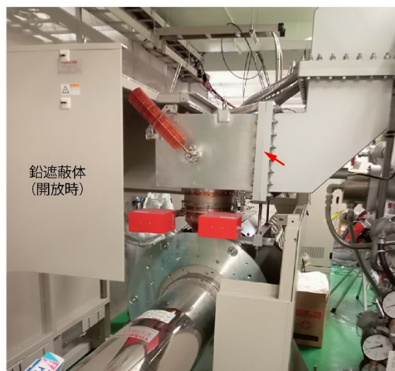
Figure 7: A photograph of a leakage point of the RF at the connection of the rectangle waveguide at the output of the klystron. The leakage point is indicated by a red arrow.
