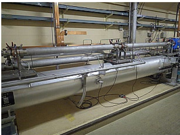
Figure 6: State of cable connection in the tunnel.
