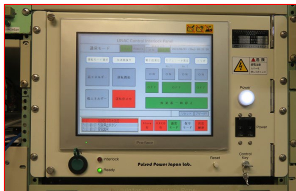
Figure 8: New operation panel (Red: Button of temporary shutdown of accelerator).
