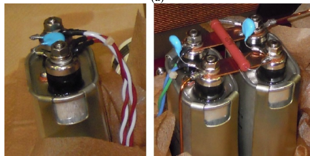
Figure 3: Capacitors that need to be exchanged in pulse transformer tanks. (a) Schematic diagram of pulse transformer tank. Three applicable capacitors are surrounded by red circles. (b) Photos of three capacitor.
