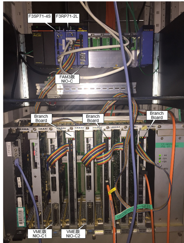
Figure 3: Comparison of NIO system based on VME (conventional system) and FA-M3 (new system). Even if using FA-M3 NIO-C, it needs to use branch board as a VME-based board.
