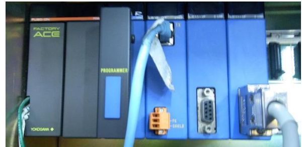
Figure 2: PLC (YOKOGAWA FA-M3).
