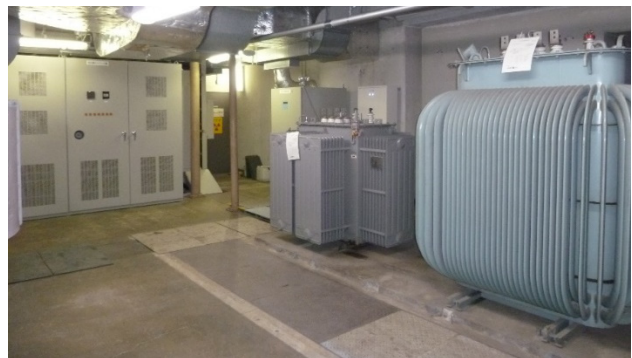
Figure 4: New power board and old transformer.
