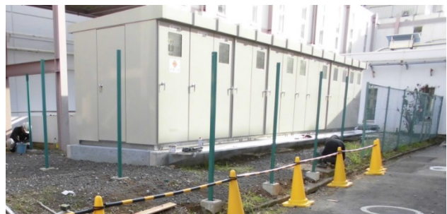
Figure 3: New transformer system for collective housings.
