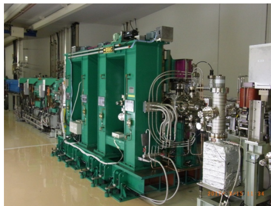
Figure 3: External view of an in-vacuum undulator after refurbishment.
