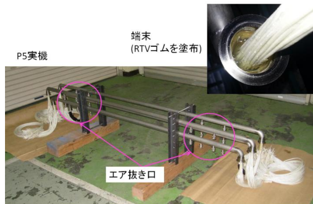
Figure 7: P5 signal cable ducts
