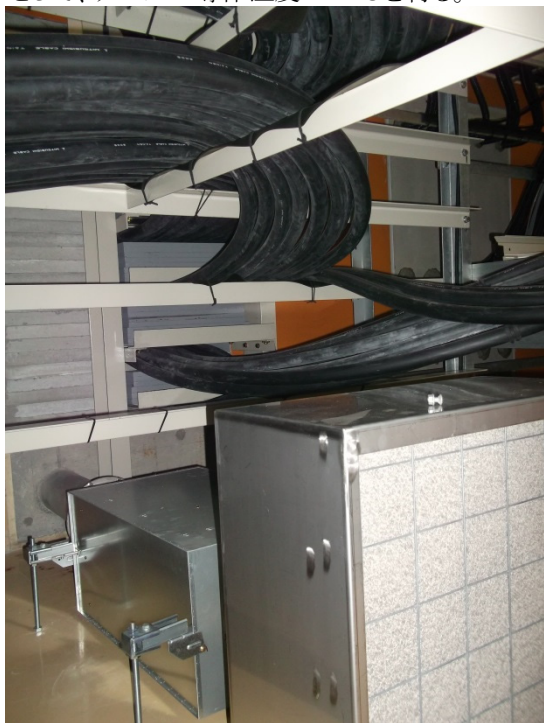
Figure 4: Cable cooling system with FDF.
