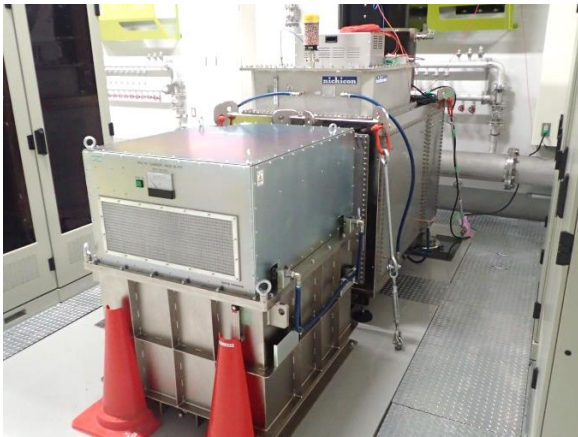
Figure 4: (Upper) PFN charger: type I, and (Lower) type II with the klystron-modulator installed in SACLA-BL1 linac.
