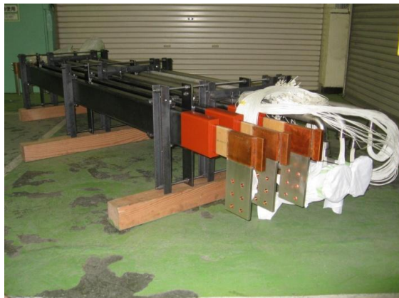
Figure 9: P6 utility duct (signal cable ducts, electric power bus ducts, water pipes, a vacuum pipe)
