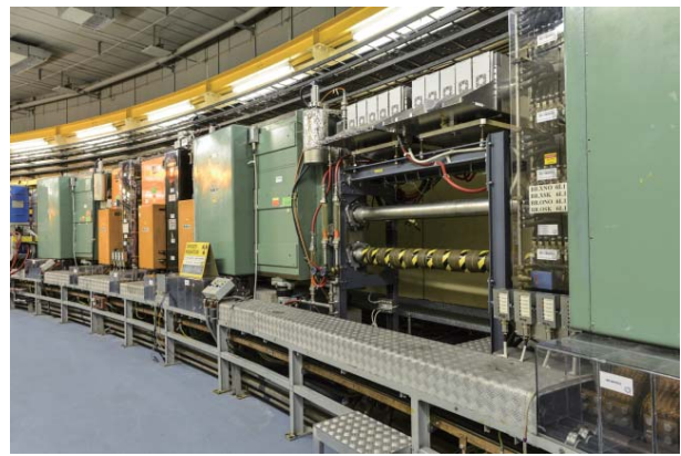
Figure 2: FT3L cavities were installed in PSB.
