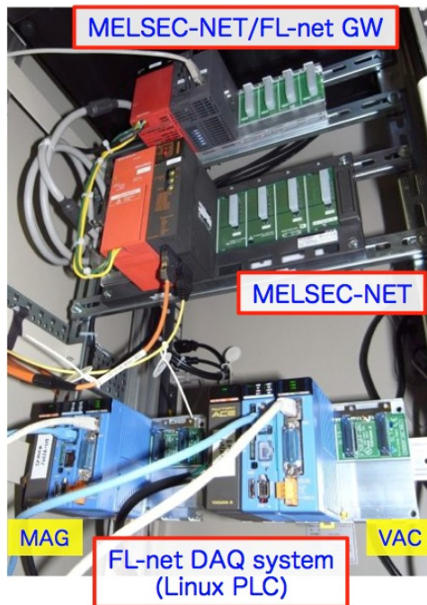
Figure 3: Data acquisition system for the vacuum and magnet protection interlock system at slave 25 rack.
