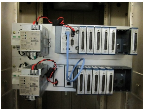
Figure 5: CompactRIO under installation. The light blue cable is used in order to interconnect the EtherCAT slave chassis (down) to the EtherCAT master controller (up).
