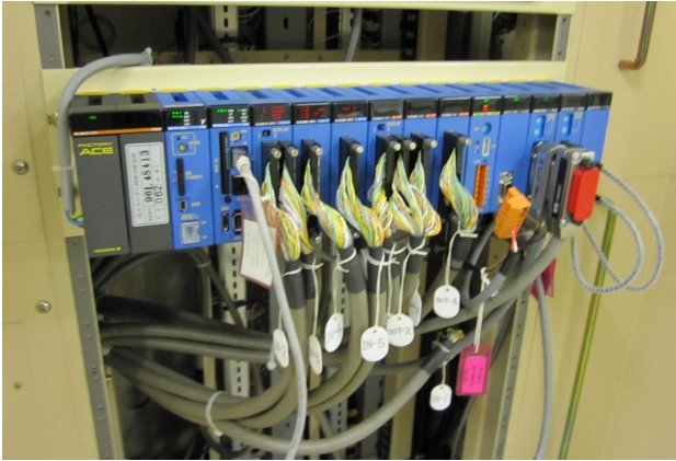
Figure 4: Consolidation of front-end computers. Left most is a power supply module (double width). Next to its right is an ordinary CPU module which runs ladder programs. Next to its right is the F3RP61 CPU module which functions as an IOC.
