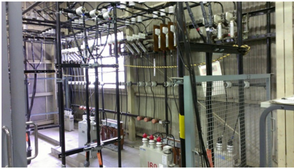
Figure 10: Newly built automatic power factor regulator.
