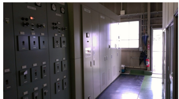
Figure 9: Relocated transformers for klystron modulators and cooling systems from the radiation controlled area.
