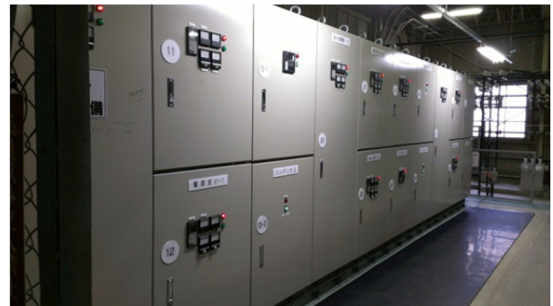
Figure 8: Renewed relays and circuit breakers.
