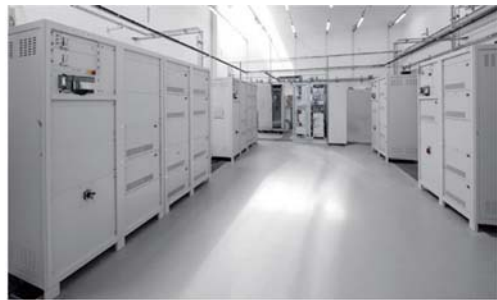
SOLEIL (Saclay – FRANCE) Ramped PSU, 3 Hz pseudo-sinus output for booster ring, 450 V/250 A 1000 V/560 A, 4 quadrants, secondary Switch mode for dipoles, quadrupoles and sextupoles magnets
