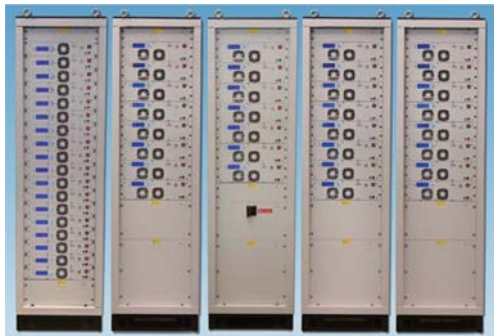
ForschungsZentrum Julich (GERMANY) PSU for beam transport based on our standard 2-5-11 kW product line, Keyboard, LCD display, USB and Ethernet port on each unit
